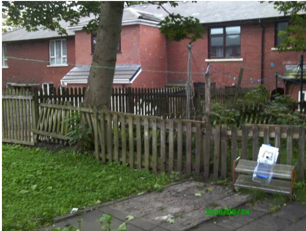
Example of poor rear fencing
